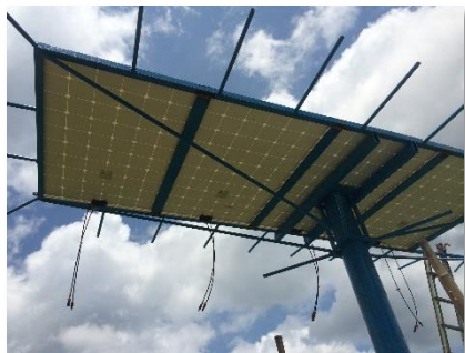
Figure 5 - Installed Solar PV at LAC facility (Source: Authors)
