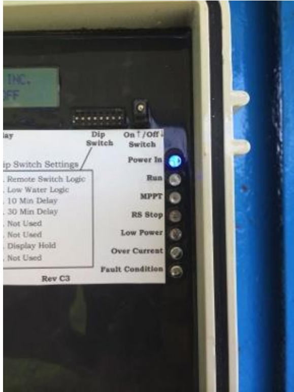
Figure 6. Image of the LED lights on the control box
