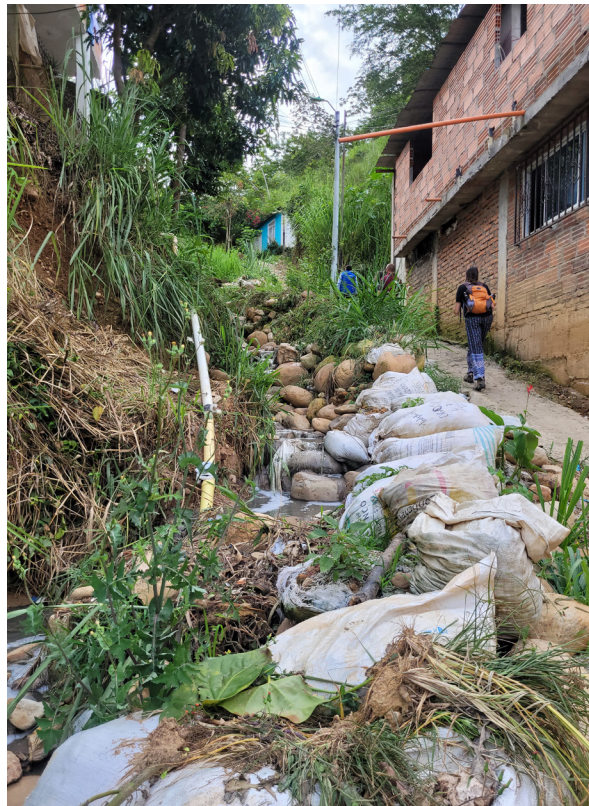
Image 4: Photo of an area that had recently experienced a mudslide and the current water infrastructure.
