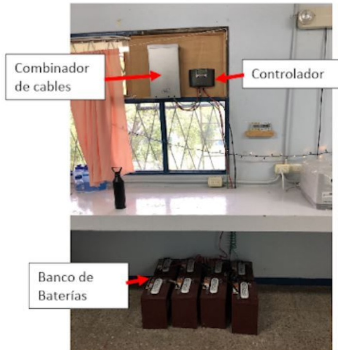
Figure 2. Photo of Combination Box, Controller, and 8 Lithium Ion Batteries.
