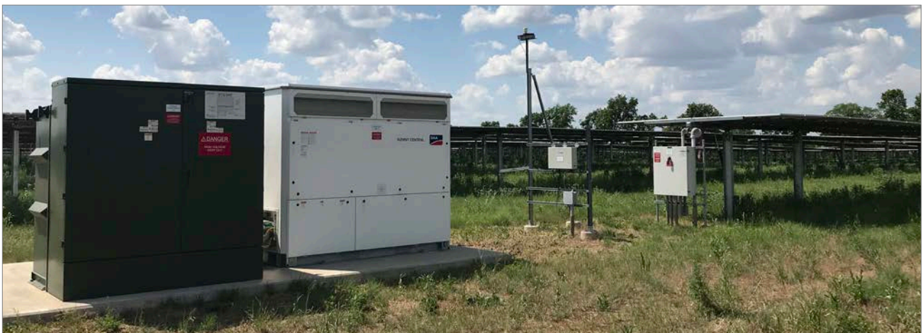
Noise sources like inverters may be staked before concrete is poured. Photo by Mary Reilly.
