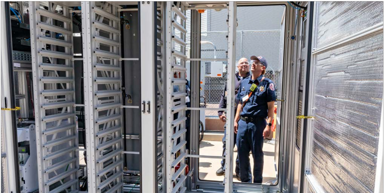
Emergency and fire response planning are especially critical for battery energy storage systems. Photo by Werner Slocum / NREL 68385.
