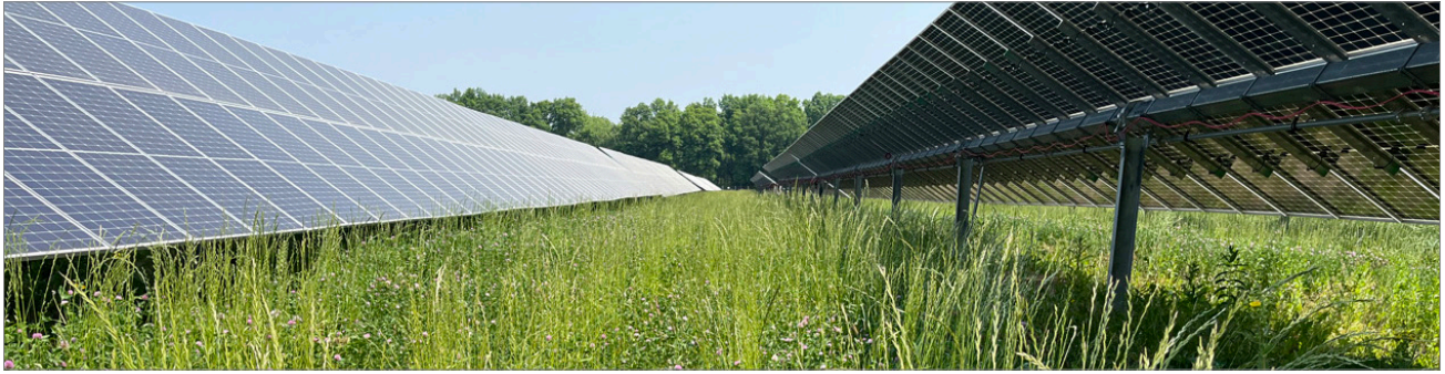
Established groundcover below solar panels at Calhoun Solar in Calhoun County. Photo by Invenergy.
