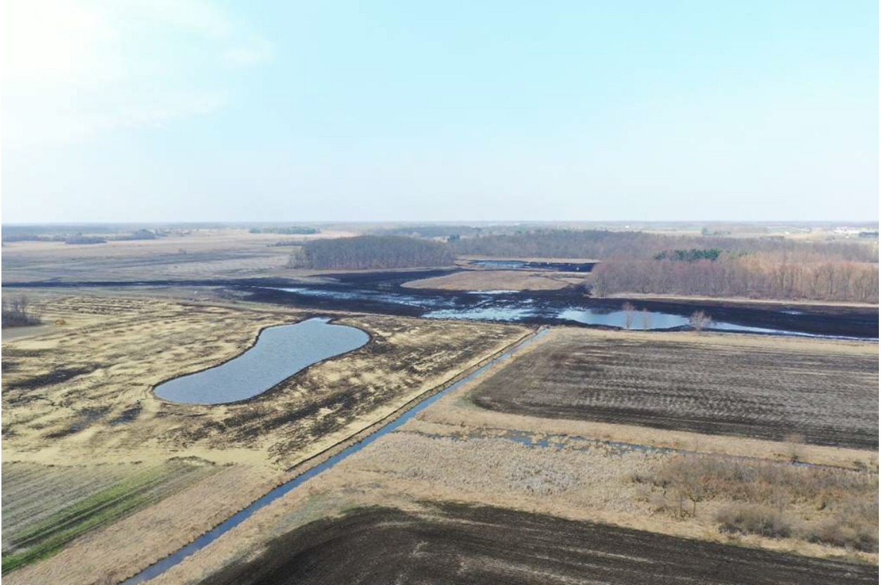
Phase I restoration began in late 2025 for the Western Lake Erie Basin pilot wetland restoration project at the Seneca State Game Area in Lenawee County, MI, USA.
