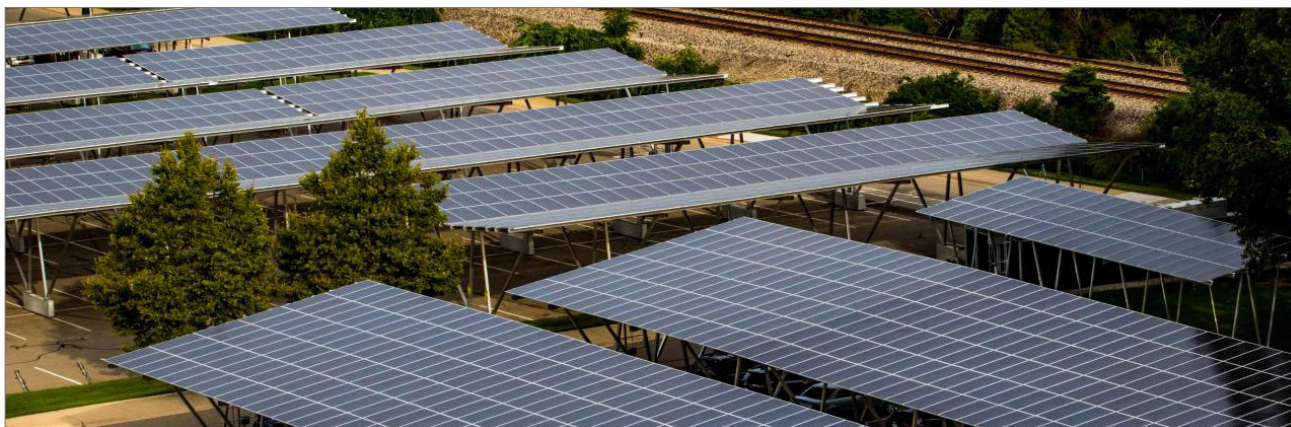
Michigan State University Solar Carport, located in East Lansing. Photo by Michigan State University.
