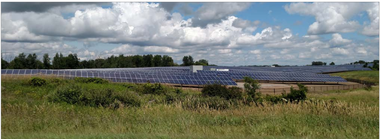
Lapeer Solar Farm, located on municipal land. Photo by Brad Neumann.
