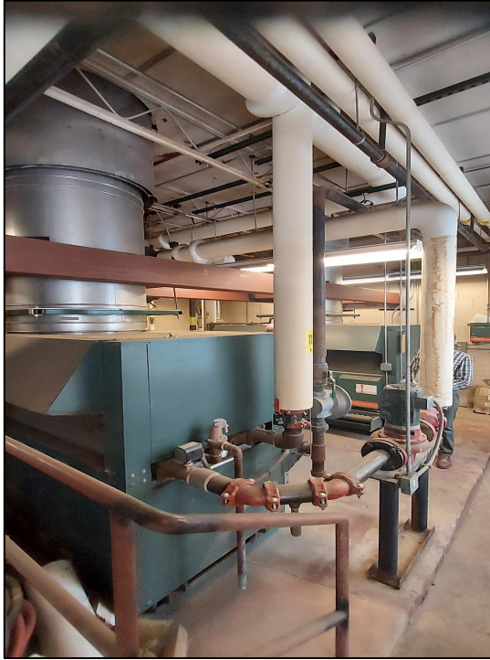
Current boilers have 2-3 years left of use
