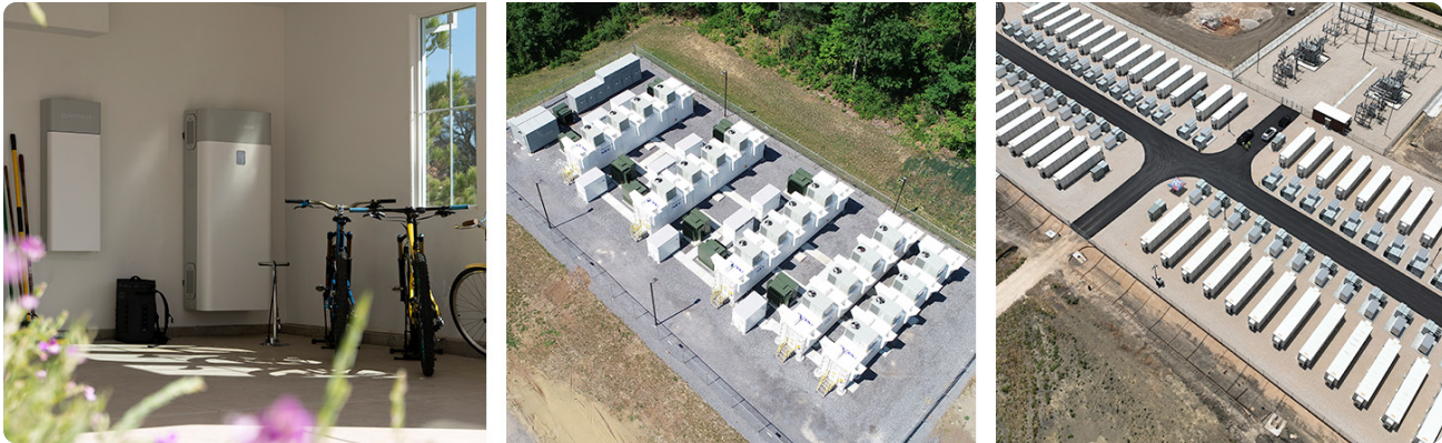
BESS at various scales: A residential on-site BESS, a small off-site BESS with 20 MW in New York, and a large off-site BESS with 100 MW in Texas. (Photos: SunPower; Key Capture Energy)
