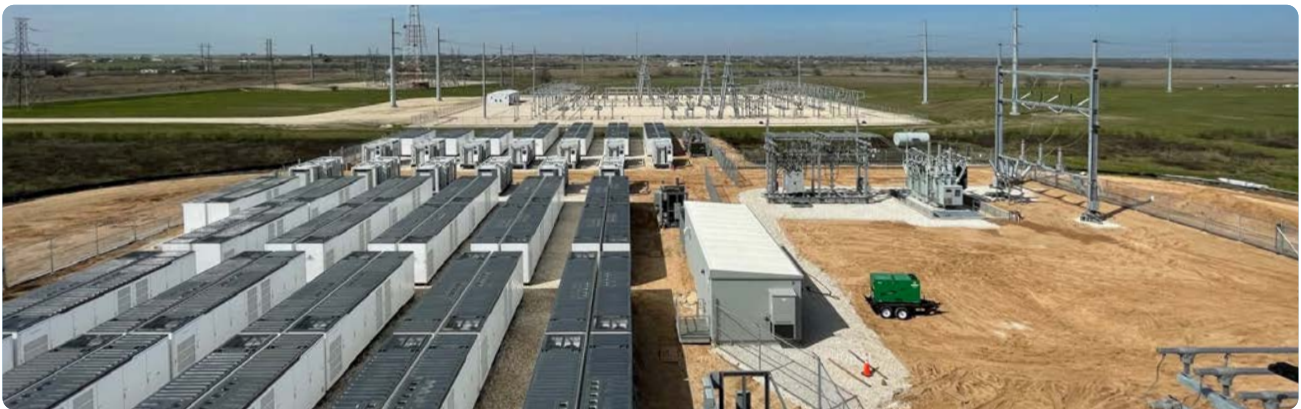
Two 50 MW BESS under construction in Texas, with a transmission substation in the background and a project substation on the right. (Photo: Key Capture Energy)
