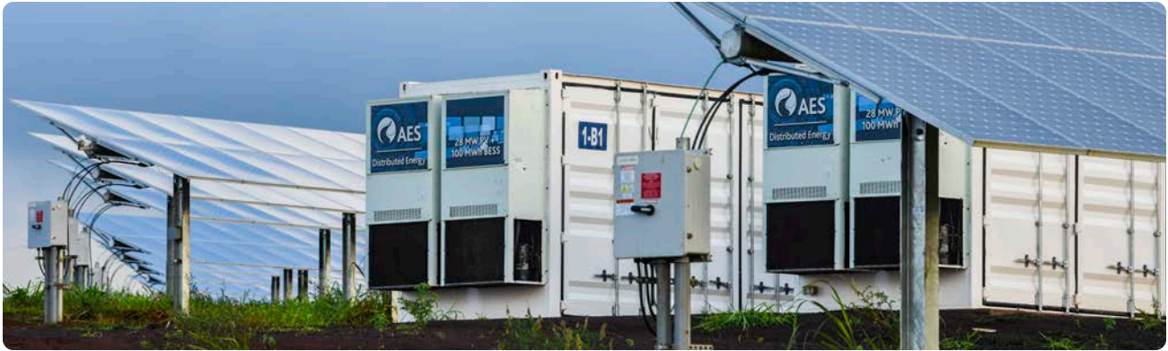
The AES Lawai Solar Project pairs BESS with solar photovoltaic energy to increase grid reliability and energy independence on Kaua’i Island, HI (Photo: Dennis Schroeder / NREL 57997)
