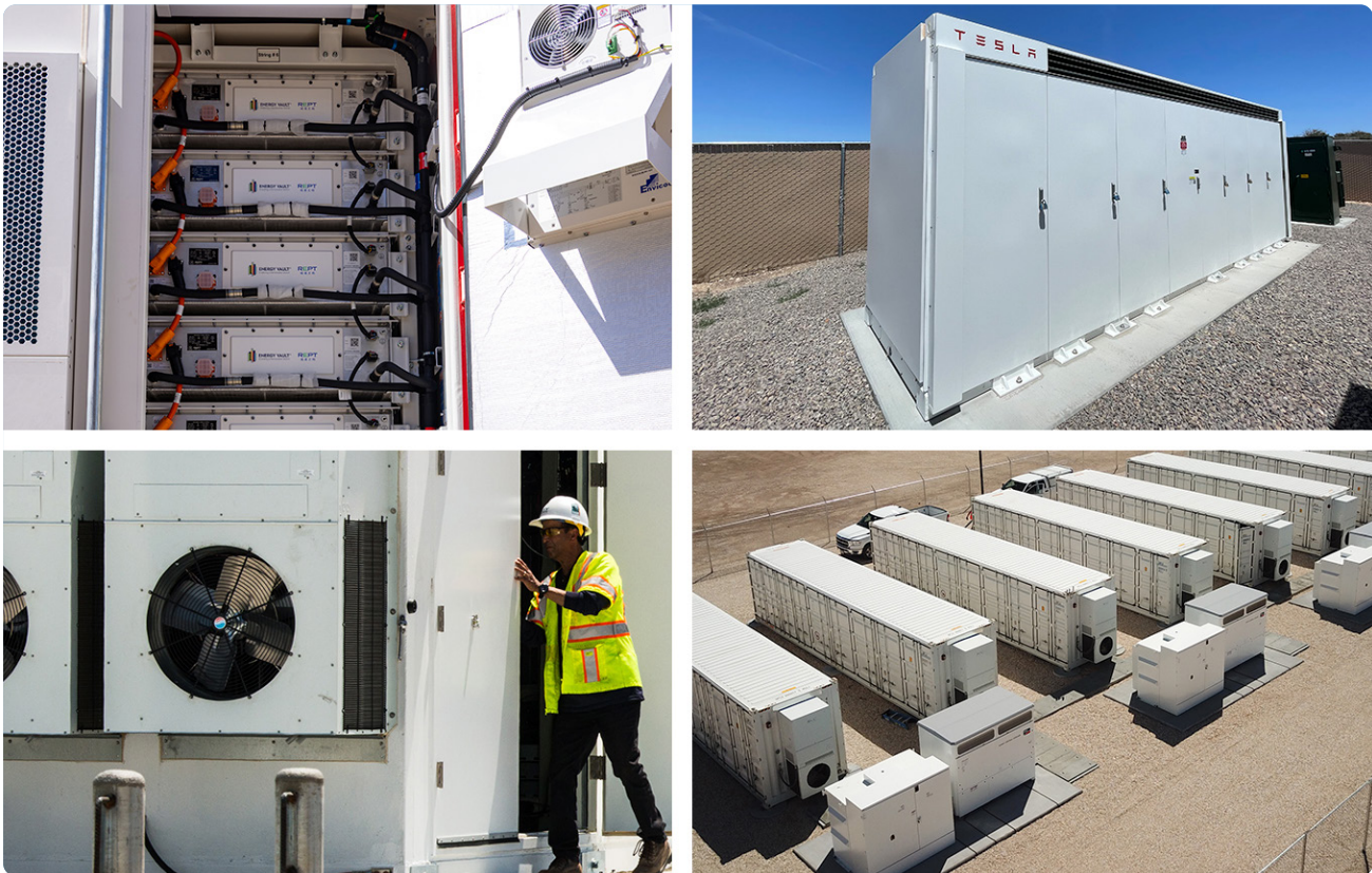
(Clockwise from top left) Battery modules (Photo: Agata Bogucka / NREL 88687); Battery enclosure (Photo: Laura Beshilas / NREL 88842); Enclosures, inverters, and transformers (Photo: Key Capture Energy); Thermal management system (Photo: Dennis Schroeder / NREL 50688)
