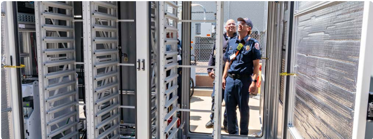
Fire fighters look over a battery cabinet during on-site training for first responders learning how to respond in the event of an emergency. (Photo: Werner Slocum / NREL 68385)
