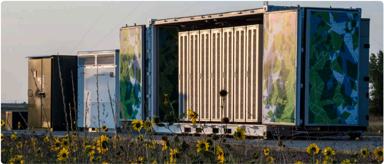
National Renewable Energy Laboratory's grid integration research facility in Colorado. (Photo: Dennis Schroeder / NREL 47220)
