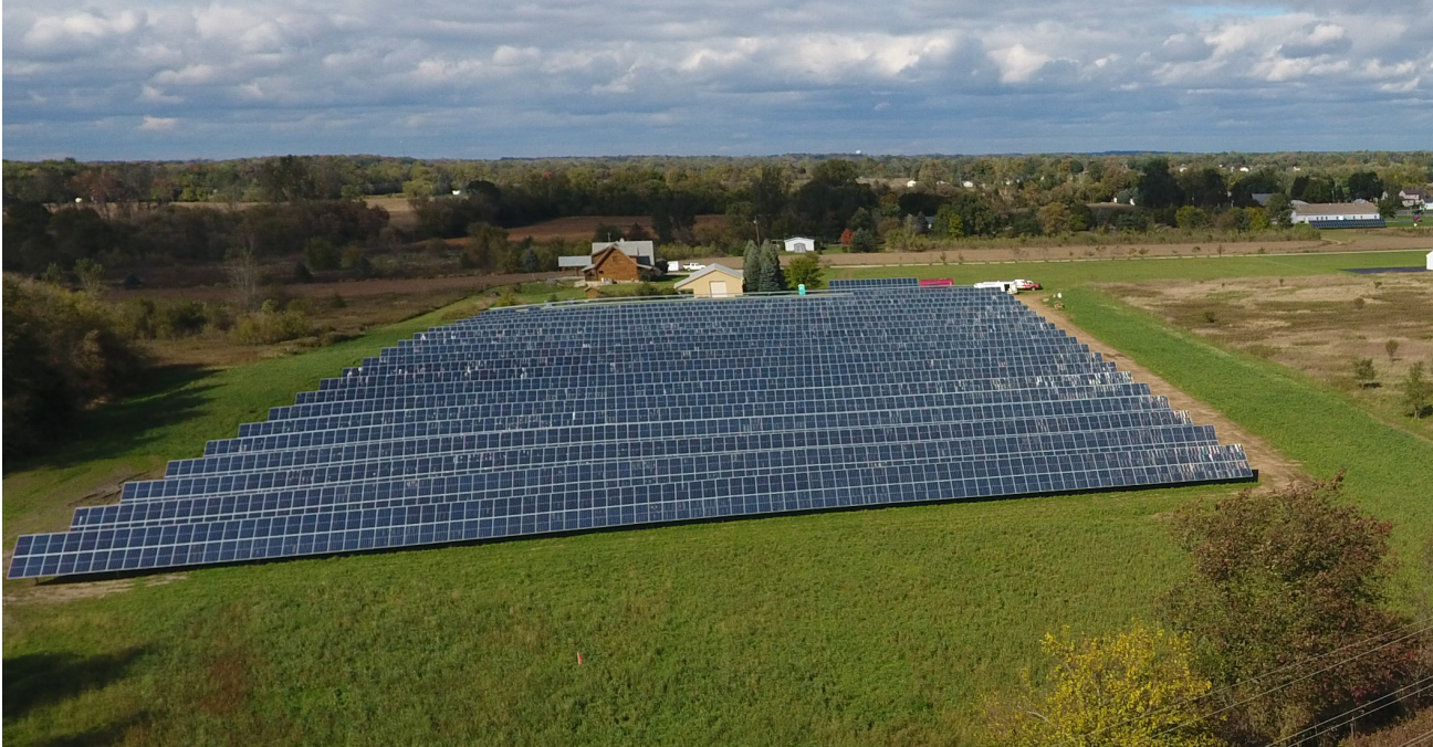
Aerial view of Tecumseh solar farm. Photo by Harvest Solar.
