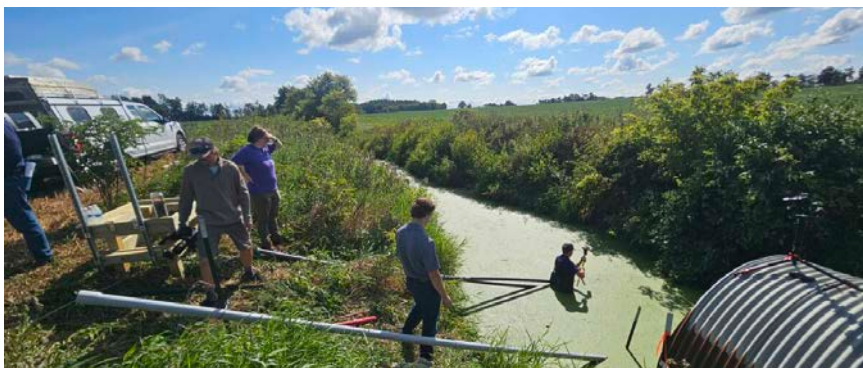
Installation of turbidity sensors near Adrian, MI. Photo: LimnoTech/Freeboard Technology.
