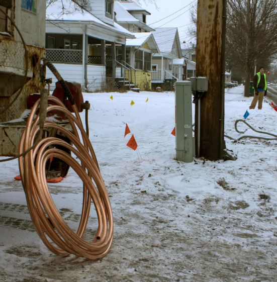
A copper service line will replace a lead service line on this residential street in Lansing. In the background is a lead service line that's been removed. Image taken and courtesy of Lindsey Scullen of Michigan Radio
